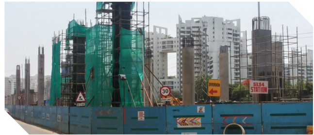
Rapid Metro Rail Gurgaon South Extension Limited (RMGSL) Gurgaon Metro Rail South Extension
